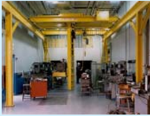
Free Standing Stacker Crane with additional Single Girder Crane
